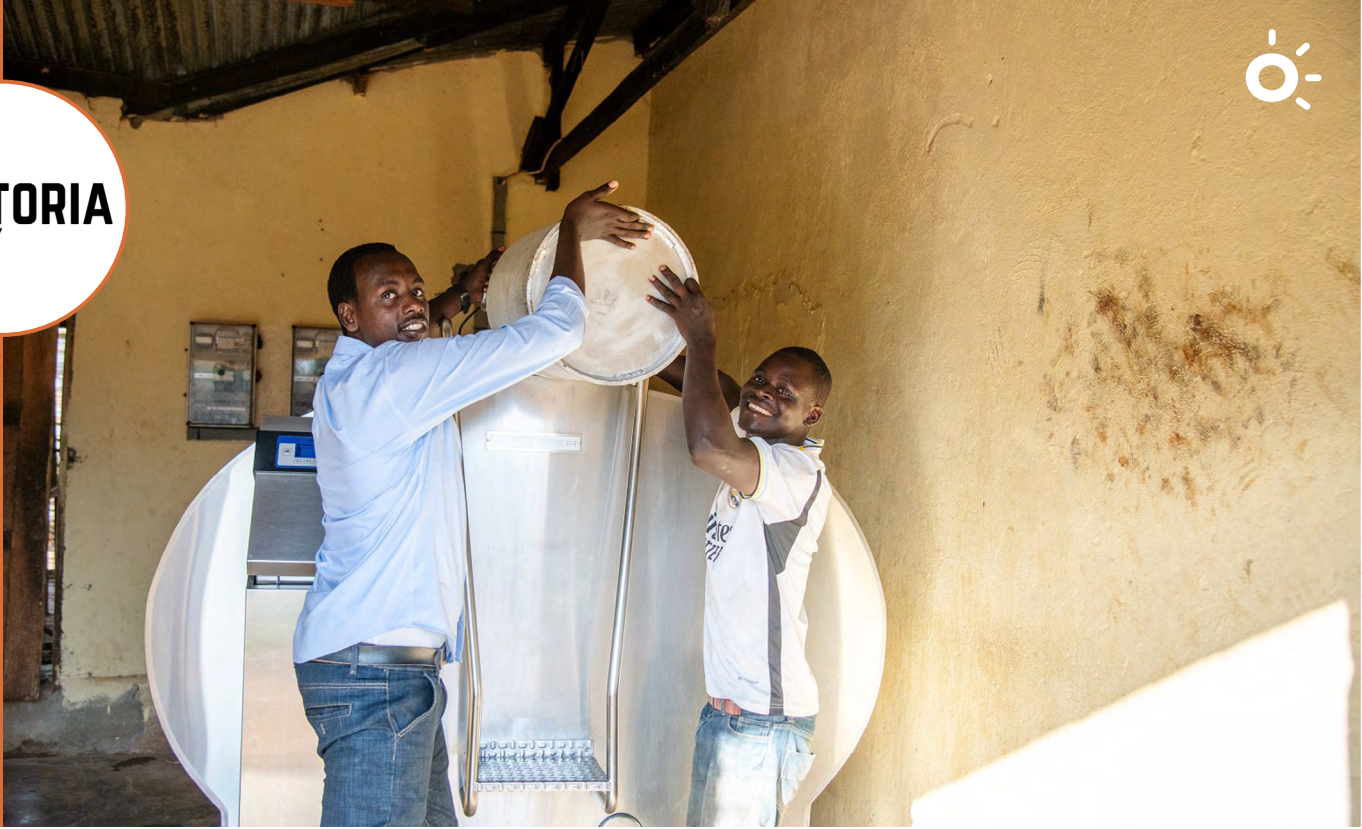
Dairy cooperatives in Southwest Uganda utilise mini-grid power from FRES Solar, a battery leasing client of Vittoria Technology (2025) Photo credit: AVSI Foundation.
