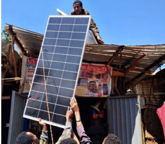
IES technicians install a second-life battery and solar-powered system to power a garment shop in Amhara (2026)
