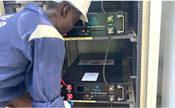
Hinckley technician commissioning a second-life battery energy storage system for a customer (2025)
