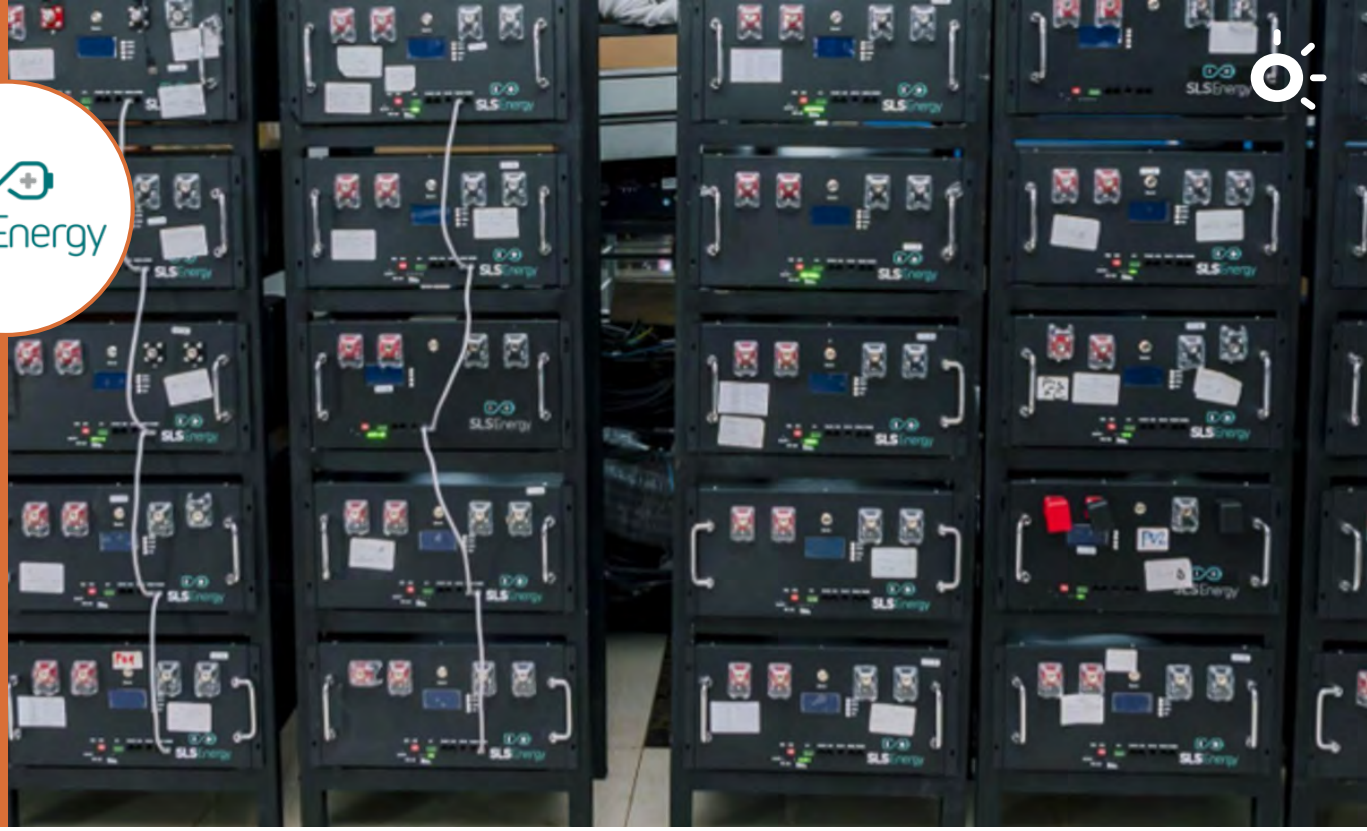
SLS battery storage system for installation at a mini-grid in Chitandika, Zambia (2026).
